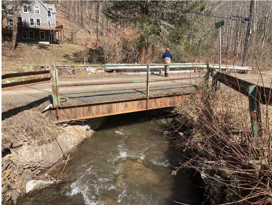
Figure 4-13: Looking downstream at the inlet of the most downstream Bonnie View Avenue at Station Road crossing over Alton Creek
