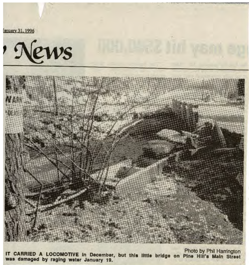
Figure 3-5: A photo depicting flood damage within the hamlet of Pine Hill on lower Main Street bridge during the January 1996 event. Photo Source: Catskill Mountain News
