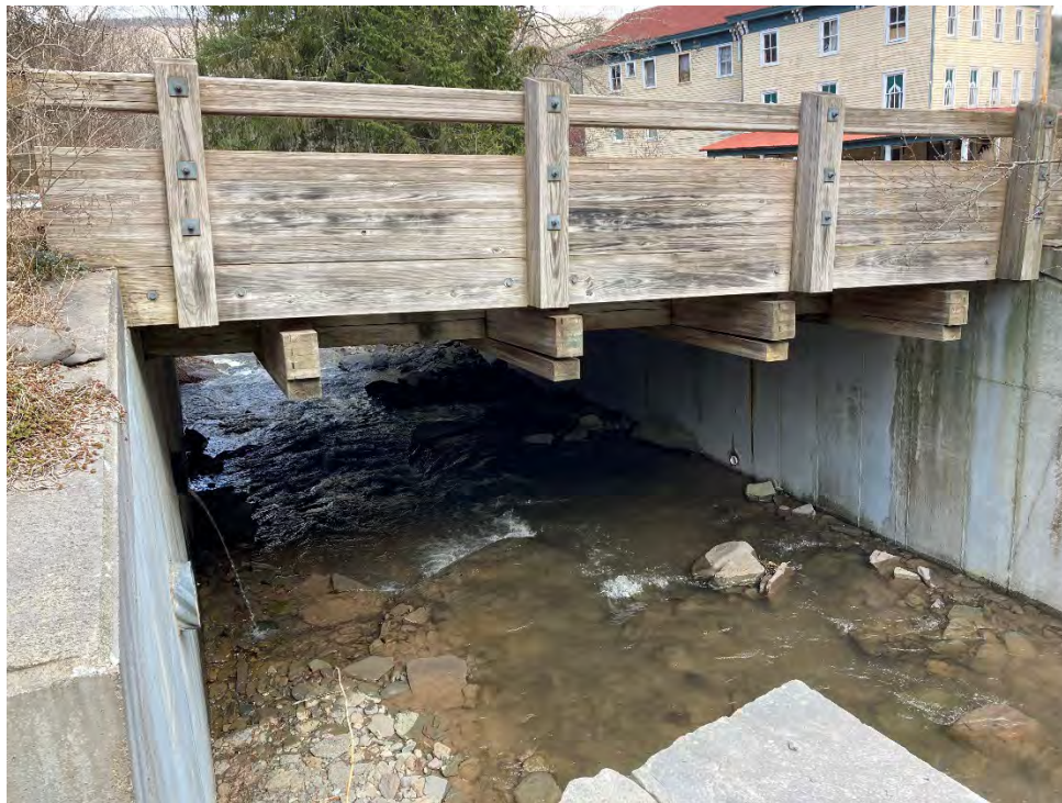
Figure 4-27: Looking downstream at the inlet of the upper Main Street crossing over Alton Creek
