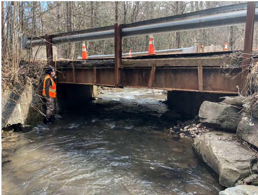
Figure 4-19: Looking downstream at the Bonnie View Avenue culvert inlet over Alton Creek
