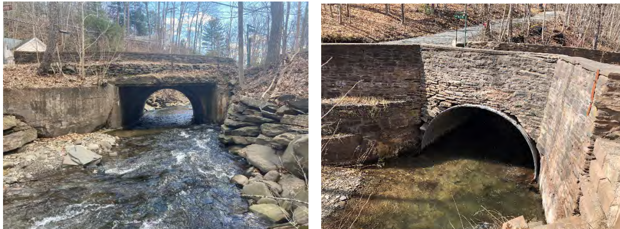
Figure 4-28: Inlet (left) and outlet (right) of Academy Street crossing over Birch Creek
