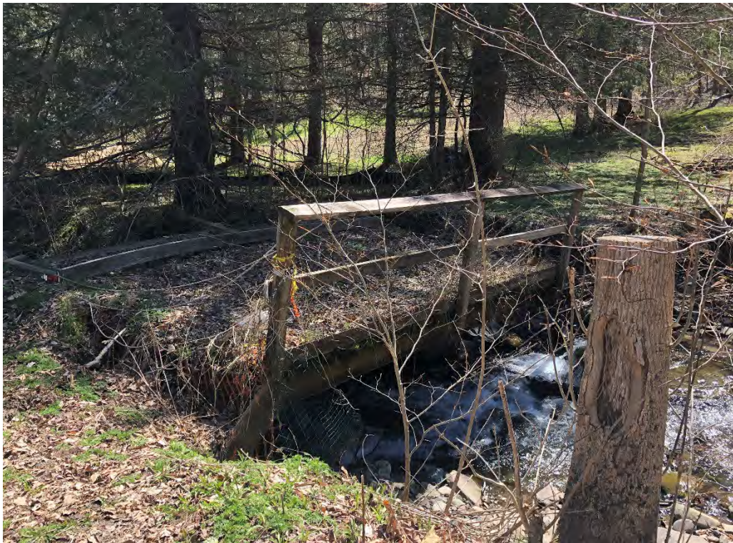
Figure 4-9: Overgrown private driveway bridge over Alton Creek
