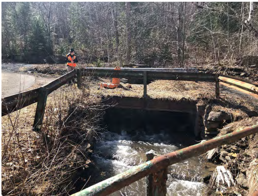
Figure 4-12: Looking upstream at the most upstream Bonnie View Avenue at Station Road crossing over Alton Creek
