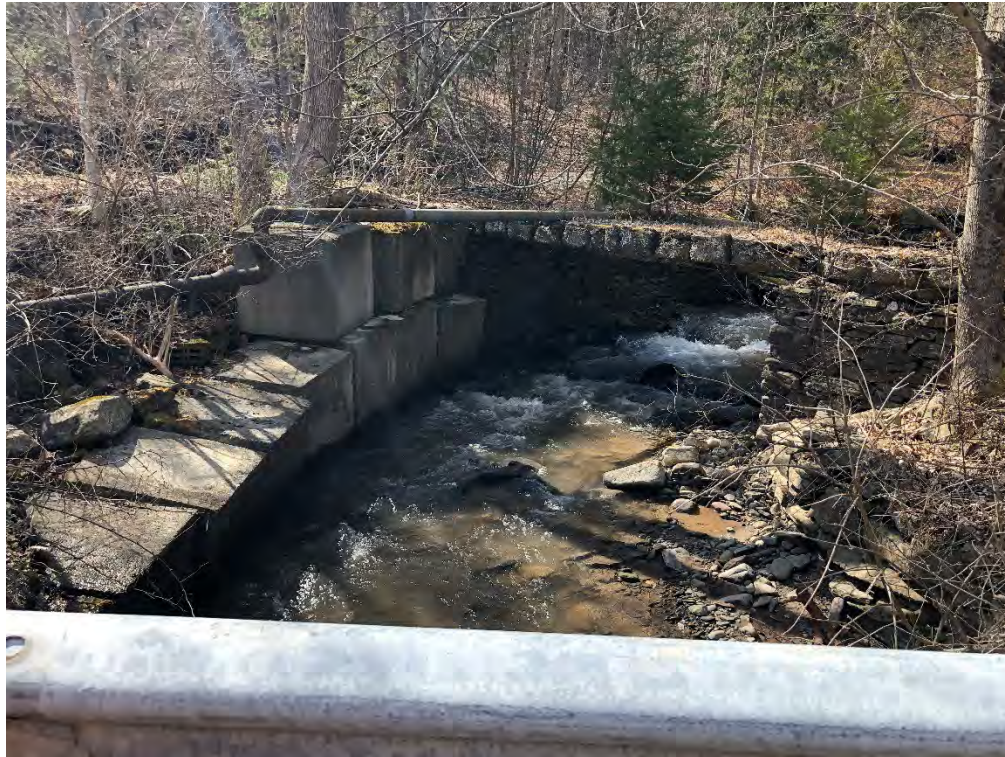
Figure 4-10: Looking upstream at stone crossing with disconnected pipe
