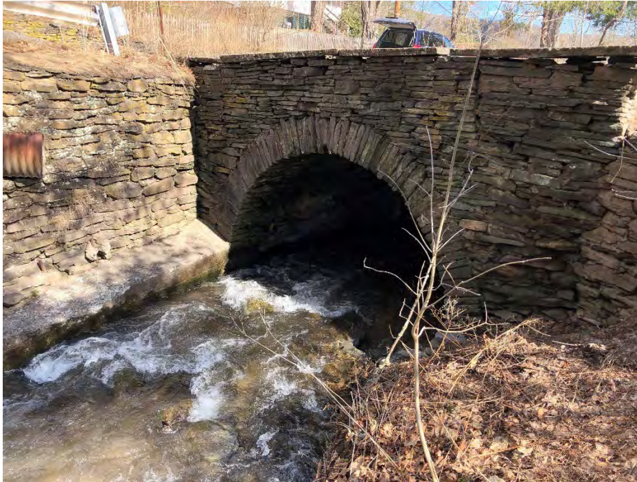
Figure 4-21: Looking downstream at the inlet of the Mill Street culvert over Alton Creek
