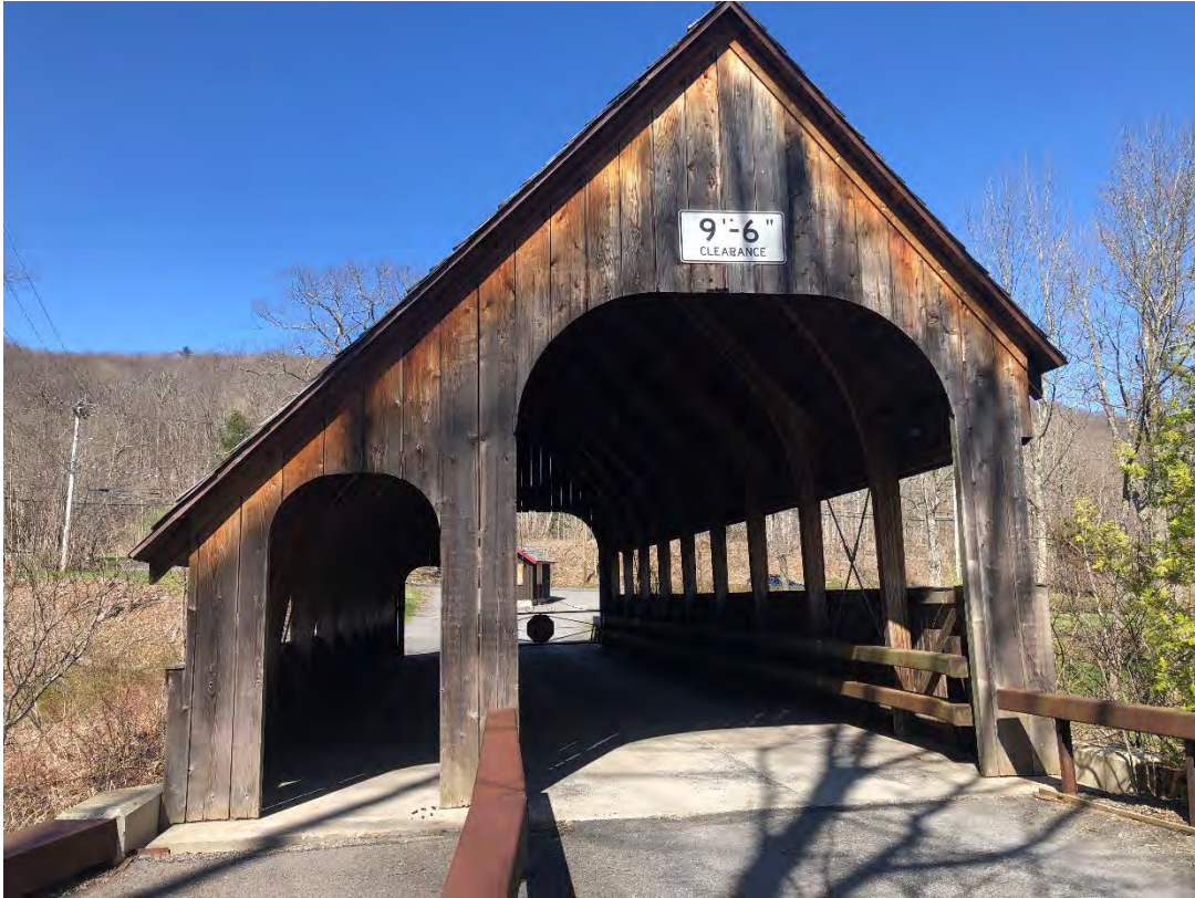
Figure 4-45: Covered bridge over Birch Creek is the only access to Belleayre Day Use Area.
