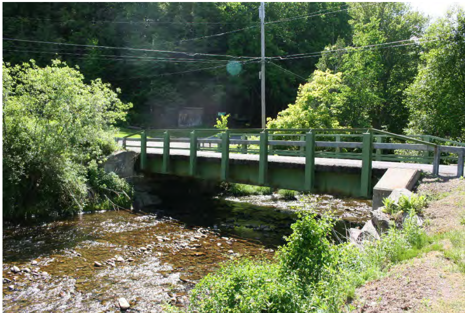
Figure 4-12: Looking upstream at the inlet of the River Road bridge over Chestnut Creek
