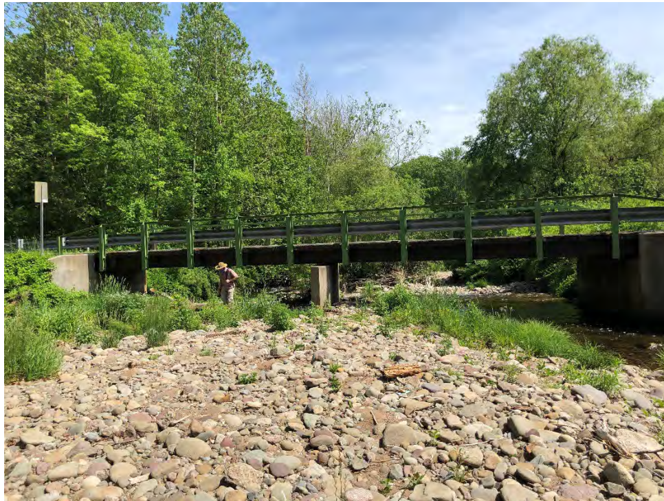
Figure 4-13: Looking downstream at the Davis Lane bridge inlet over Chestnut Creek. A prominent lateral sediment bar is located immediately upstream of the bridge.
