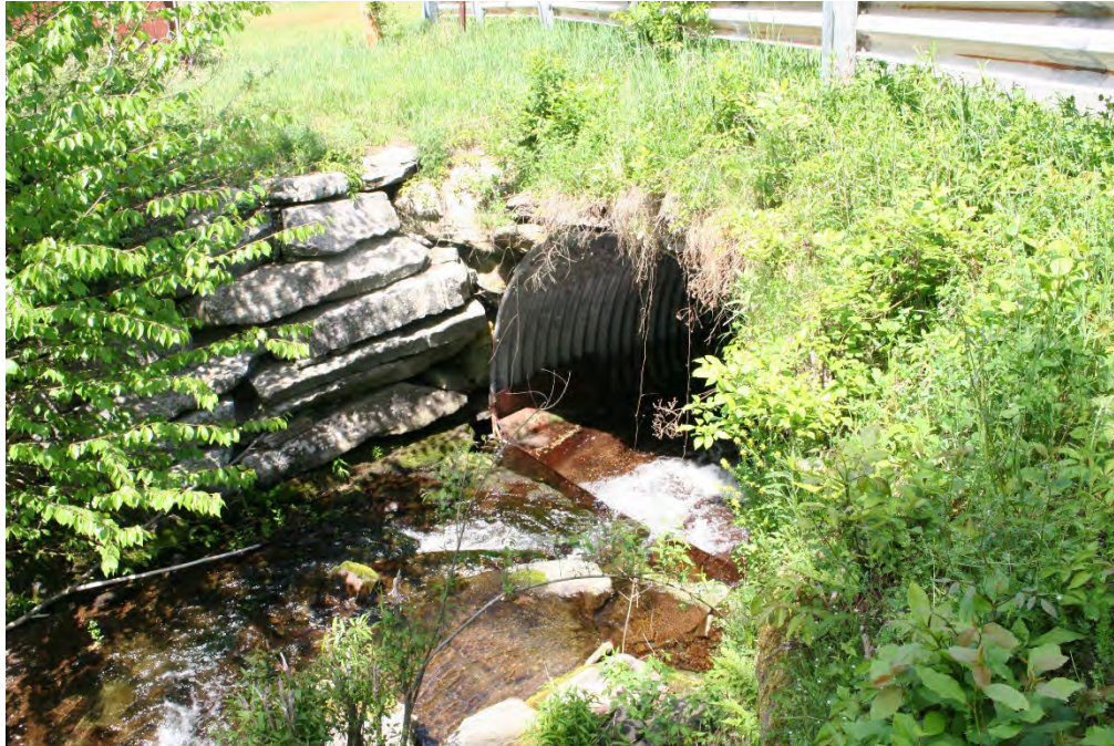
Figure 4-18: Looking downstream at Slater Road culvert over Chestnut Creek. The stacked stone wall and culvert inlet drop are also illustrated.
