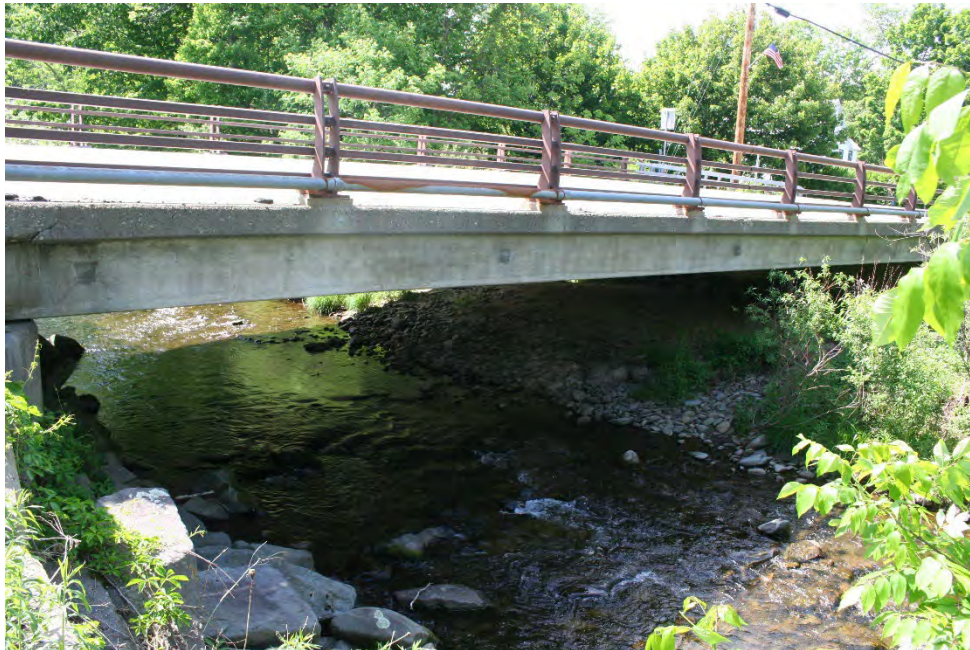
Figure 4-3: Looking upstream at the outlet of the NYS Route 42 bridge over Chestnut Creek
