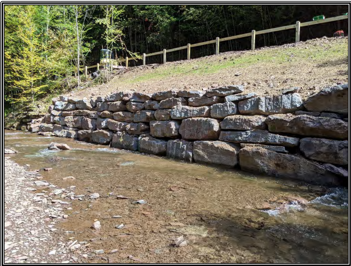
Steele Brook SL 4.52 Streambank Stabilization at Phase I, Village of Delhi, NY constructed in 2021
