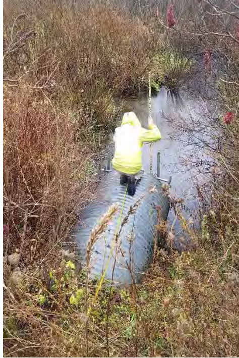
Figure 4-17: Buntline Drive culvert carrying WBDR T1 (looking downstream at projecting culvert outlet)
