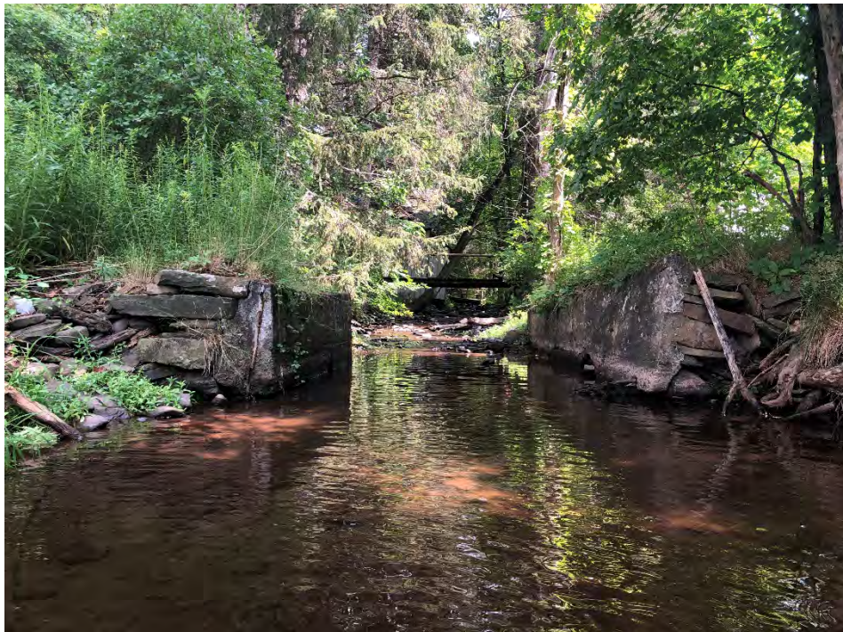
Figure 4-37: Abutment remains restricting low flows on the WBDR
