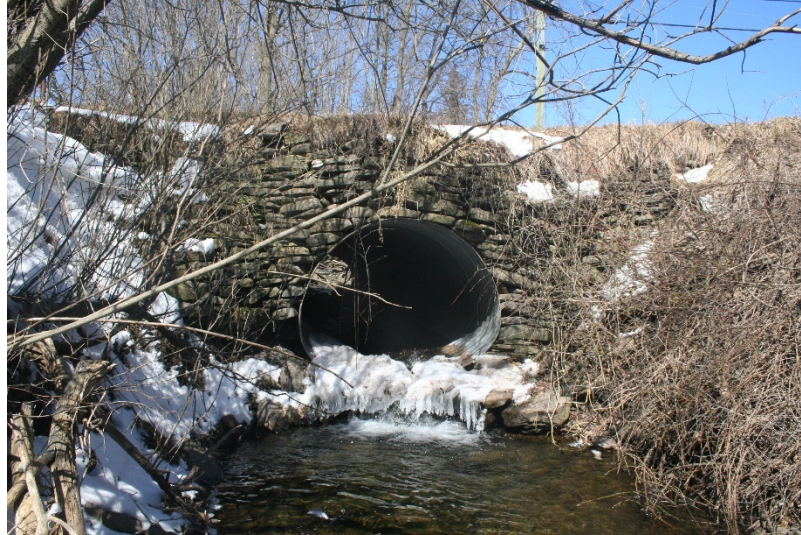
Figure 5-6: County Route 3 culvert carrying unnamed tributary. View looking upstream at culvert. Perched outlet is an impediment to aquatic organism passage and contributes to development of downstream scour hole.
