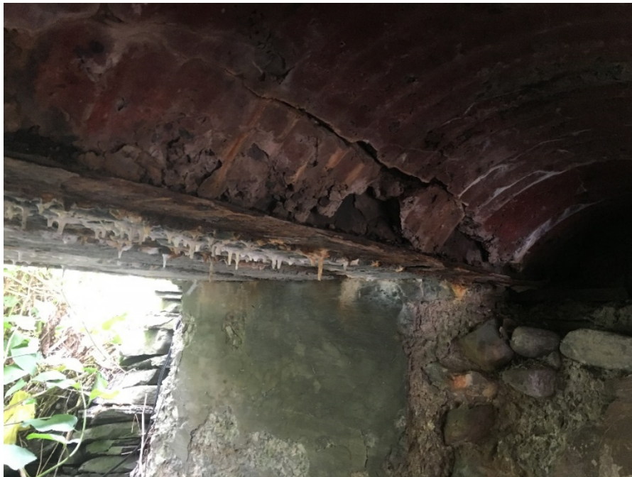
Figure 5-11: Deteriorated concrete and steel, looking at upstream left abutment. The half-pipes used as concrete forms hide the condition of the concrete where they have not yet rusted away. Note large cobbles used as aggregate in concrete abutment.
