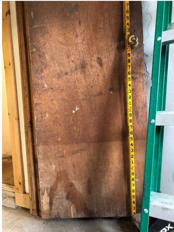
Figure 5-18: High-water mark on door inside Town Highway Garage (1.45 feet)
