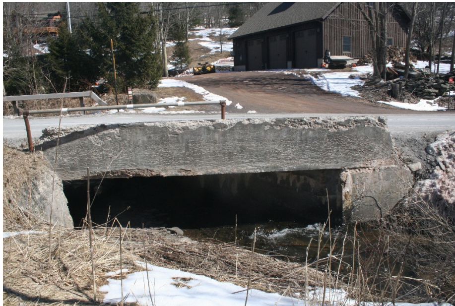
Figure 5-8: County Route 1 culvert over Brownell Creek. View from right bank, looking upstream. In floods, water flanks this culvert on the left side, flows across the driveway in the background of the image, and down the road.
