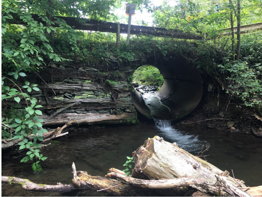
Figure 5-3: Fairbairn Drive culvert carrying Elk Creek. View looking upstream at culvert outlet. Left wingwall (right side of photograph) has failed; right wingwall (left side of photograph) is in fair condition. Perched outlet is an impediment to aquatic organism passage and may contribute to headwall failure.
