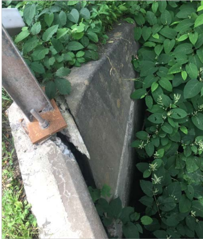
Figure 5-10: Upstream right wingwall separated from structure
