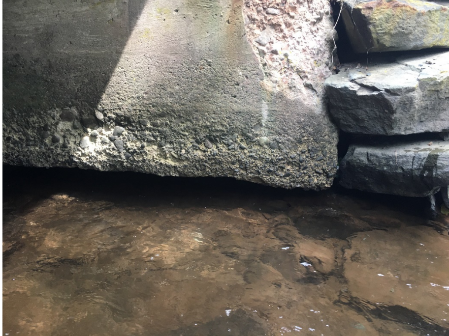
Figure 5-12: Scour has undermined several feet of the left abutment.
