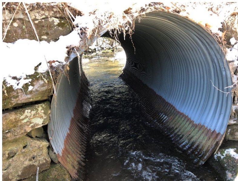
Figure 5-2: Townsend Hollow Road culvert carrying Elk Creek. View looking downstream through culvert.
