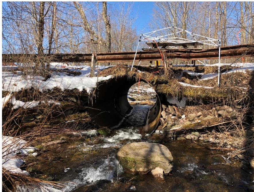
Figure 5-4: Fairbairn Drive culvert carrying Elk Creek. View looking downstream at culvert inlet. Right wingwall has failed and collapsed. Left wingwall is in poor condition. Tent frame and picnic bench cover collapsed portion of road embankment.
