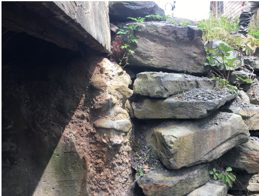
Figure 5-13: Deteriorating concrete abutment, downstream left. Note large cobbles used as aggregate in concrete.
