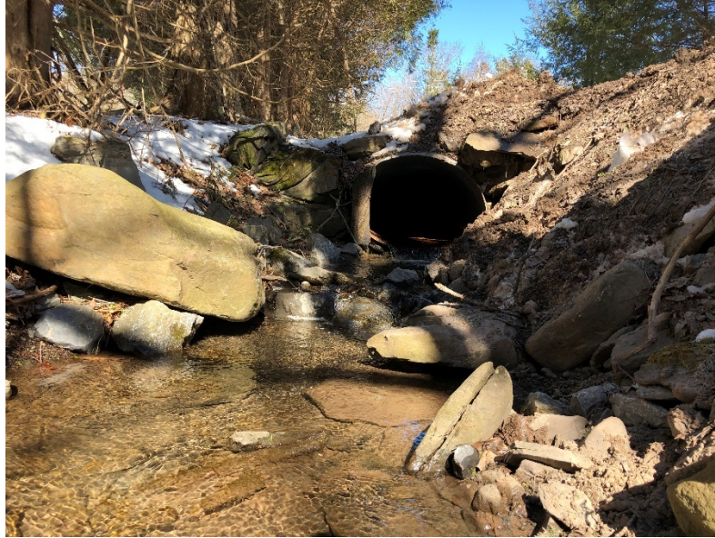
Figure 5-1: Townsend Hollow Road culvert carrying Elk Creek. View looking upstream at culvert outlet.
