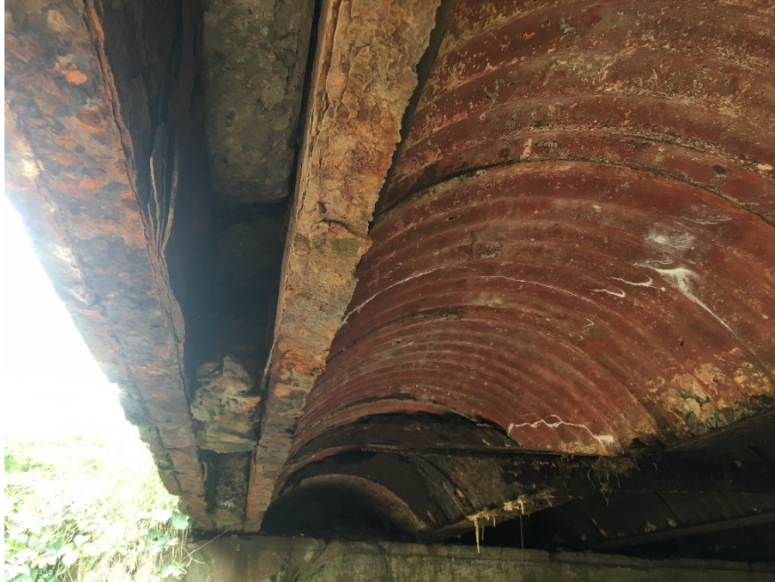
Figure 5-14: Underside of deck, looking at downstream right corner. Steel beams are rusted and exfoliating. A large amount of concrete appears to be missing from between the two beams along the left side of the image.
