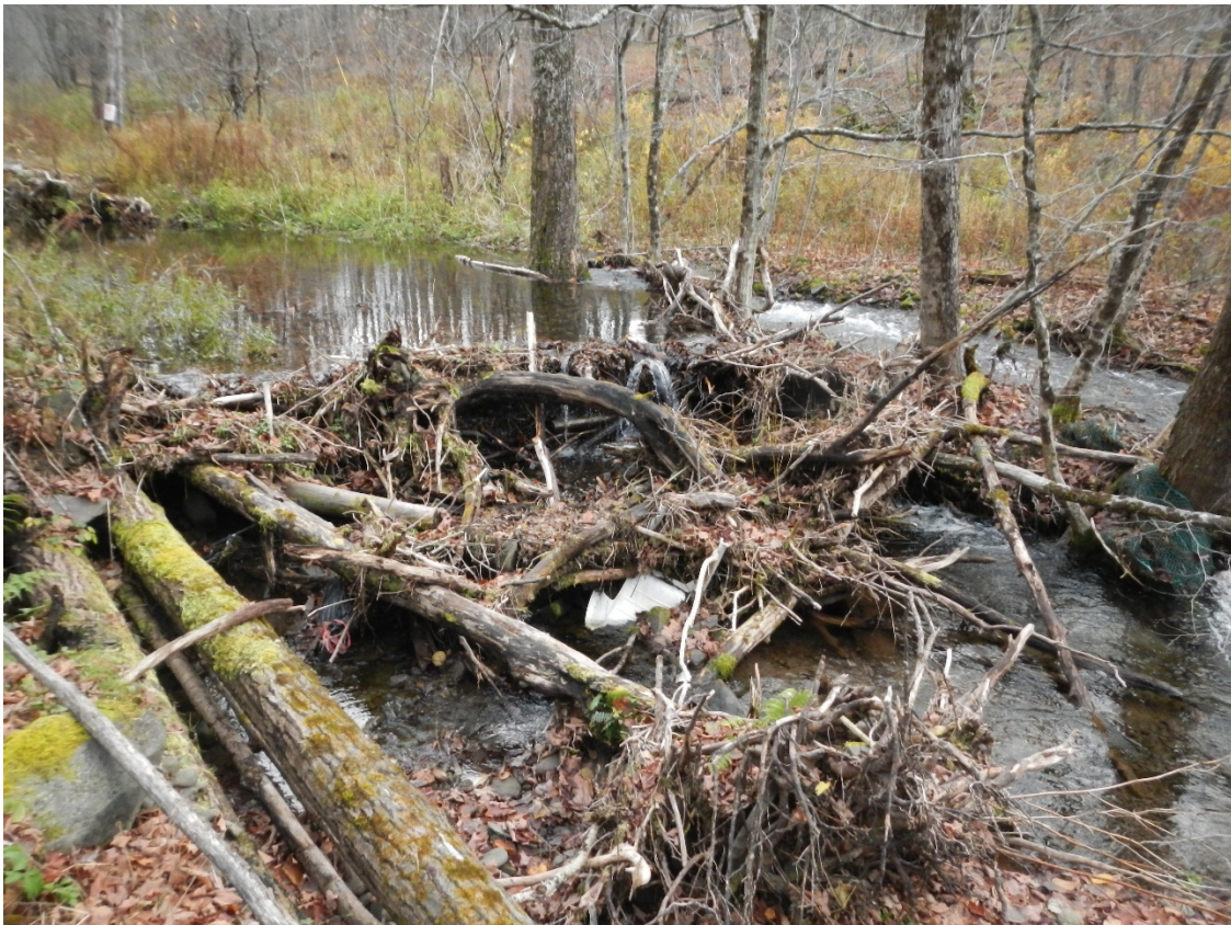
Figure 5-22: Large debris jam just downstream of Elk Creek Road bank failure.
