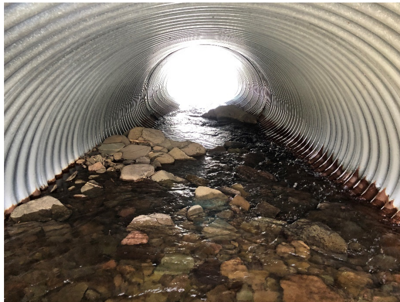
Figure 5-5: County Route 3 culvert carrying unnamed tributary. View inside culvert, looking downstream. Sediment aggradation has reduced the hydraulic capacity of the culvert.
