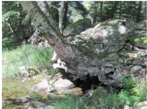
Scour on right bank downstream of berm (A235)
