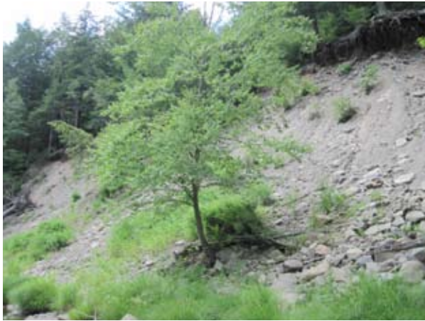
Severe slope failure on right bank (A384)
