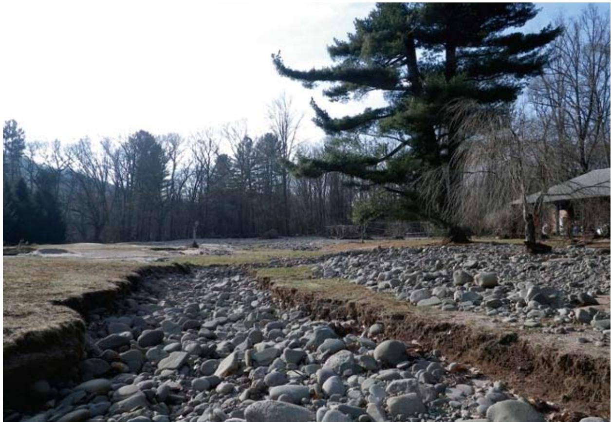
Flood chute that caused severe damage to structures in the left flood plain near Station 27800. (IMGP2327)
