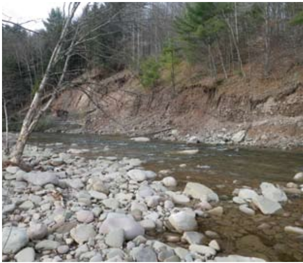
Slope failure on the right bank across from cobble point bar. (IMG1744)
