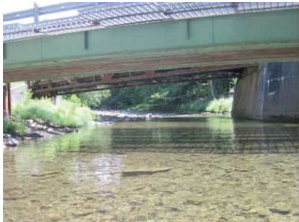
Aggradation under bridge (A326)
