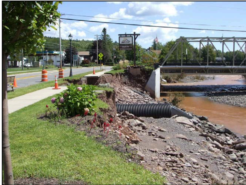
Figure 4-15 Hunter Mountain Bridge over Schoharie Creek Evidence of Erosion following Tropical Storm Irene
