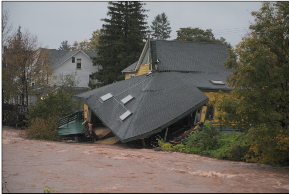
Figure 3-6 Home along Schoharie Creek Damaged by Flooding and Bank Erosion Tropical Storm Irene, August 28, 2011
