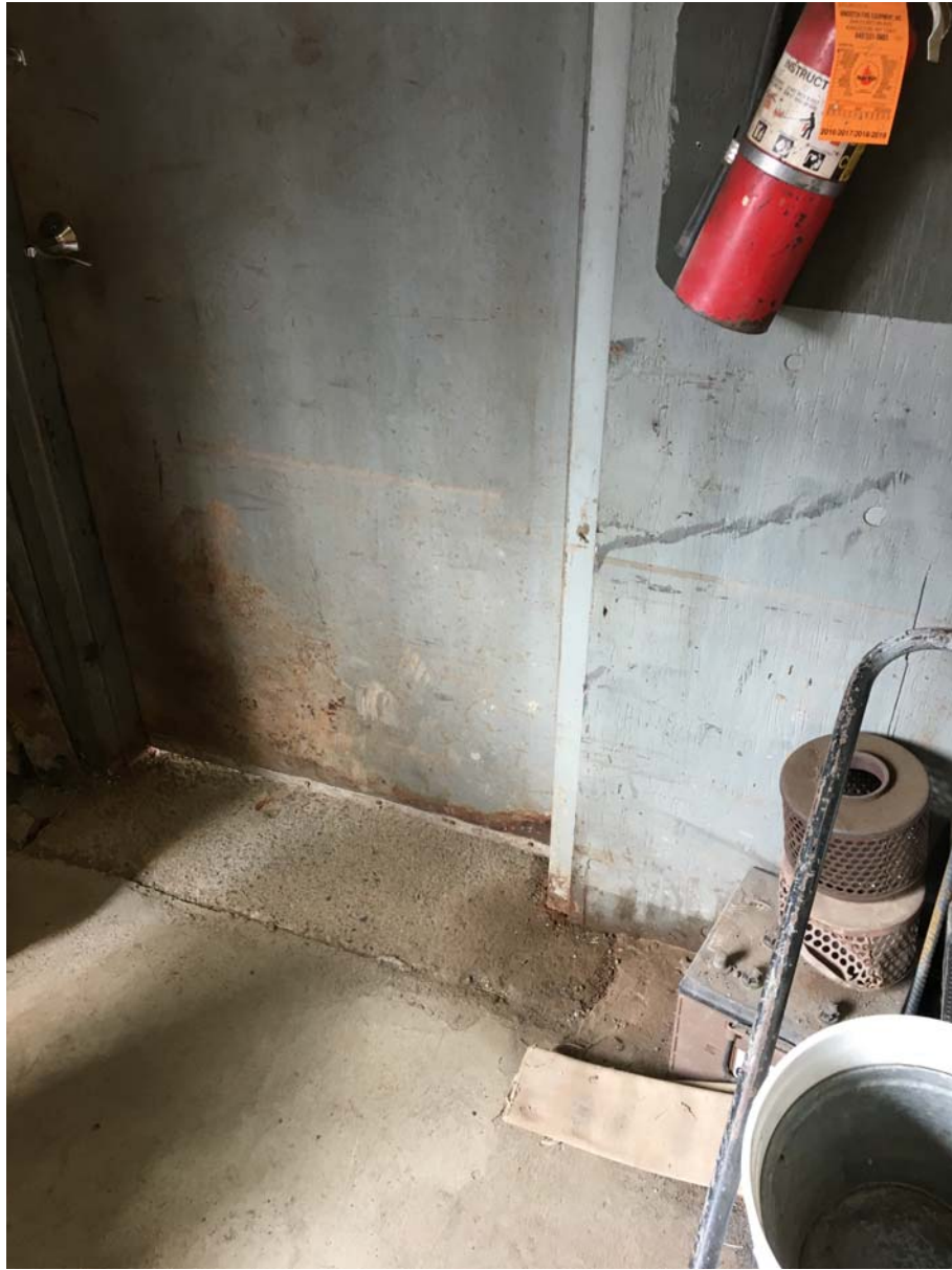
Photo #1 – Typical Water Mark on Interior of Building
