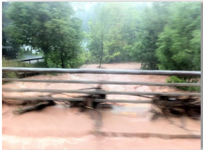
Figure 4-3 Main Street Bridge over Sawmill Creek overtopping in Tropical Storm Irene
