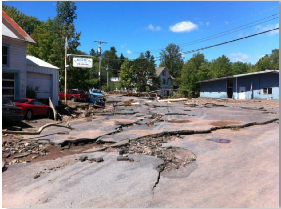
Figure 4-25 Tannersville Highway Department Garage following Tropical Storm Irene
