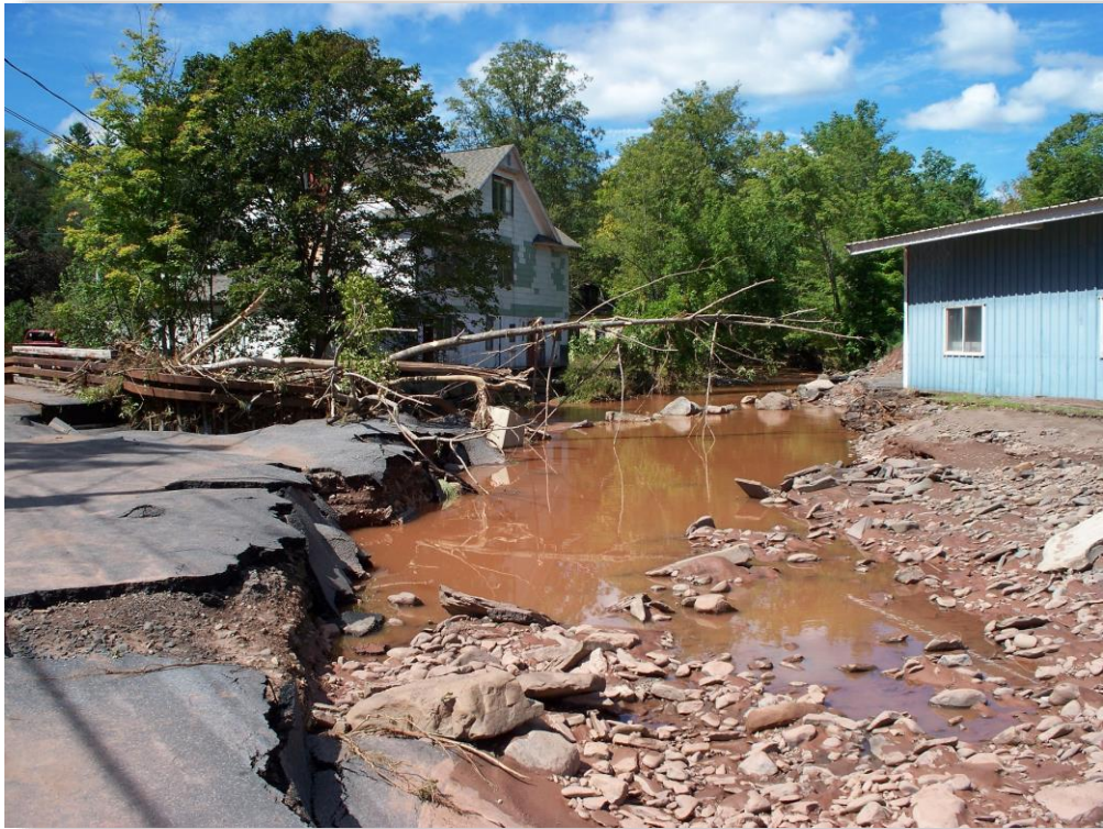
Figure 3-4 View of the Railroad Avenue bridge on the left and the DPW garage on the right the day after the flood
