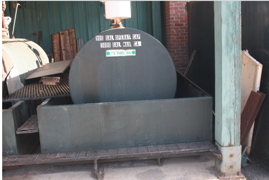
Figure 2-10 1000-gallon Fuel Storage Tank at Highway Department Garage
