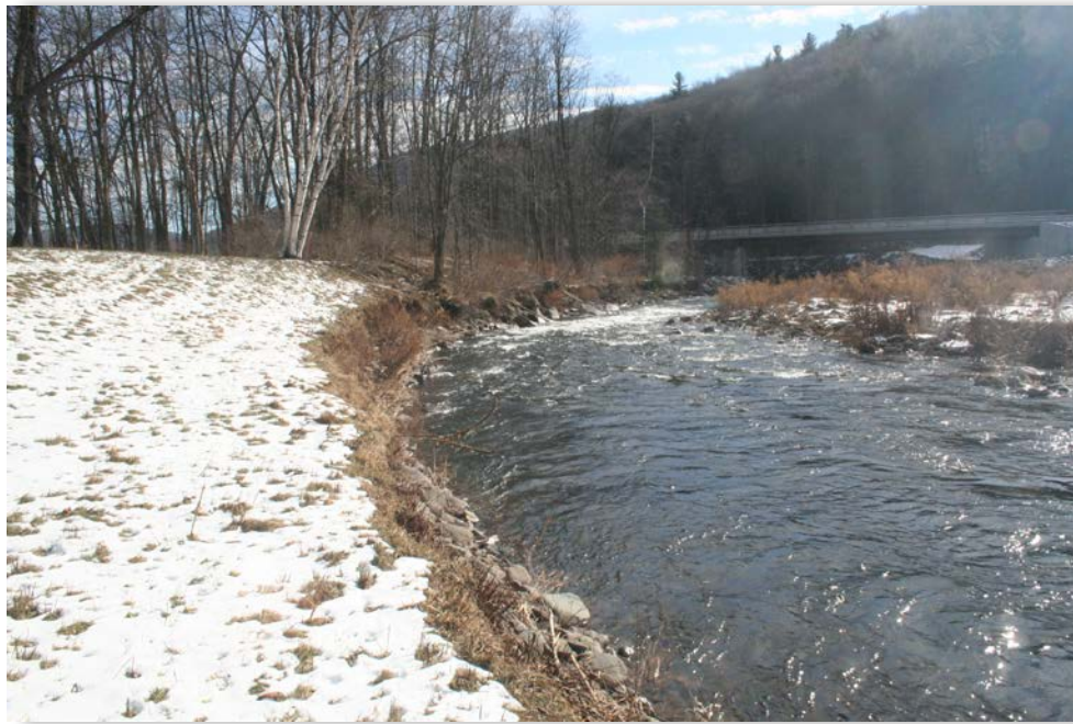
Figure 2-8 Erosion along Flood Control Levee in Shandaken
