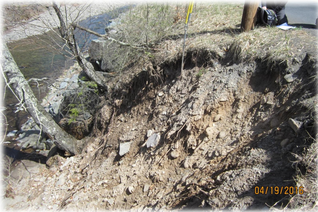
Excessive force of Rondout Creek led to erosion of bank near Peekamoose Road. Bank Repair made by the Town during the study period. (Photo 2)
