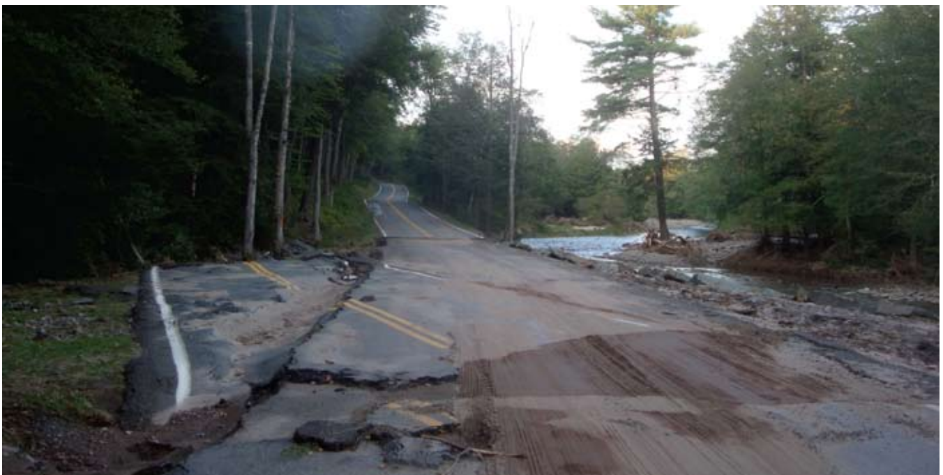
Floods cause repeated damage to County Road 47; this photo August 2011.
