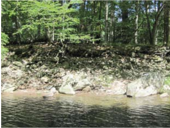
Erosion on left bank (B319)
