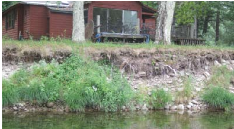
Erosion on left bank (B406)
