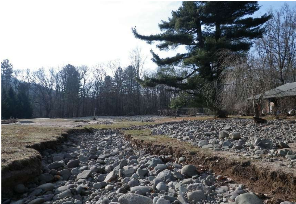
Flood chute that caused severe damage to structures in the left flood plain near Station 27800. (IMGP2327)
