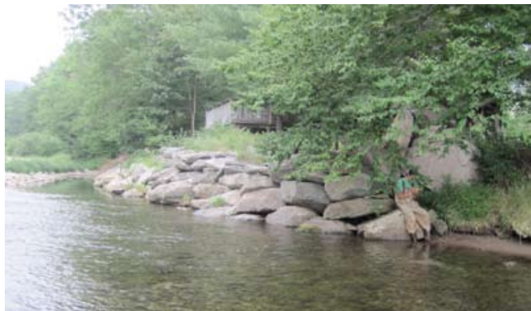
Erosion at downstream end of large revetment on left bank (B400)
