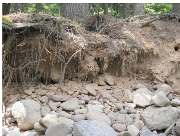
Eroding bank segment downstream of revetment (A191)
