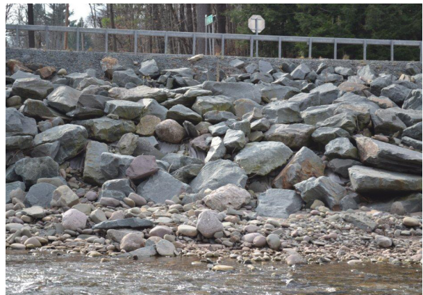
Failing rip rap, Nov. 12, 2012
