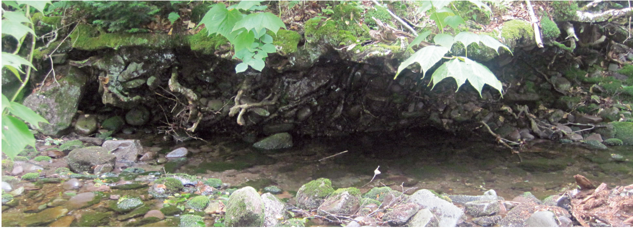
Eroding bank segment (B621)
