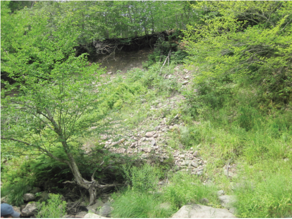
Bank failure on right bank of side channel (A1000)
