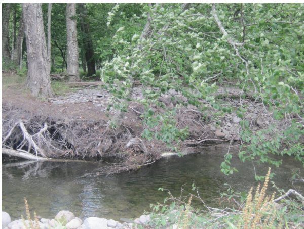
Hydraulic erosion of bank (B992)
