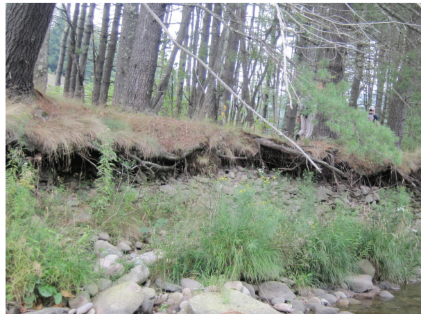
Eroding segment on left bank (B361)
