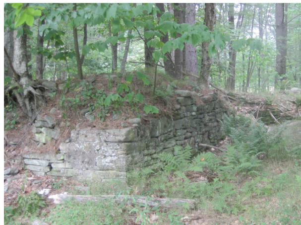
Toppled foundation on left bank (B367)
