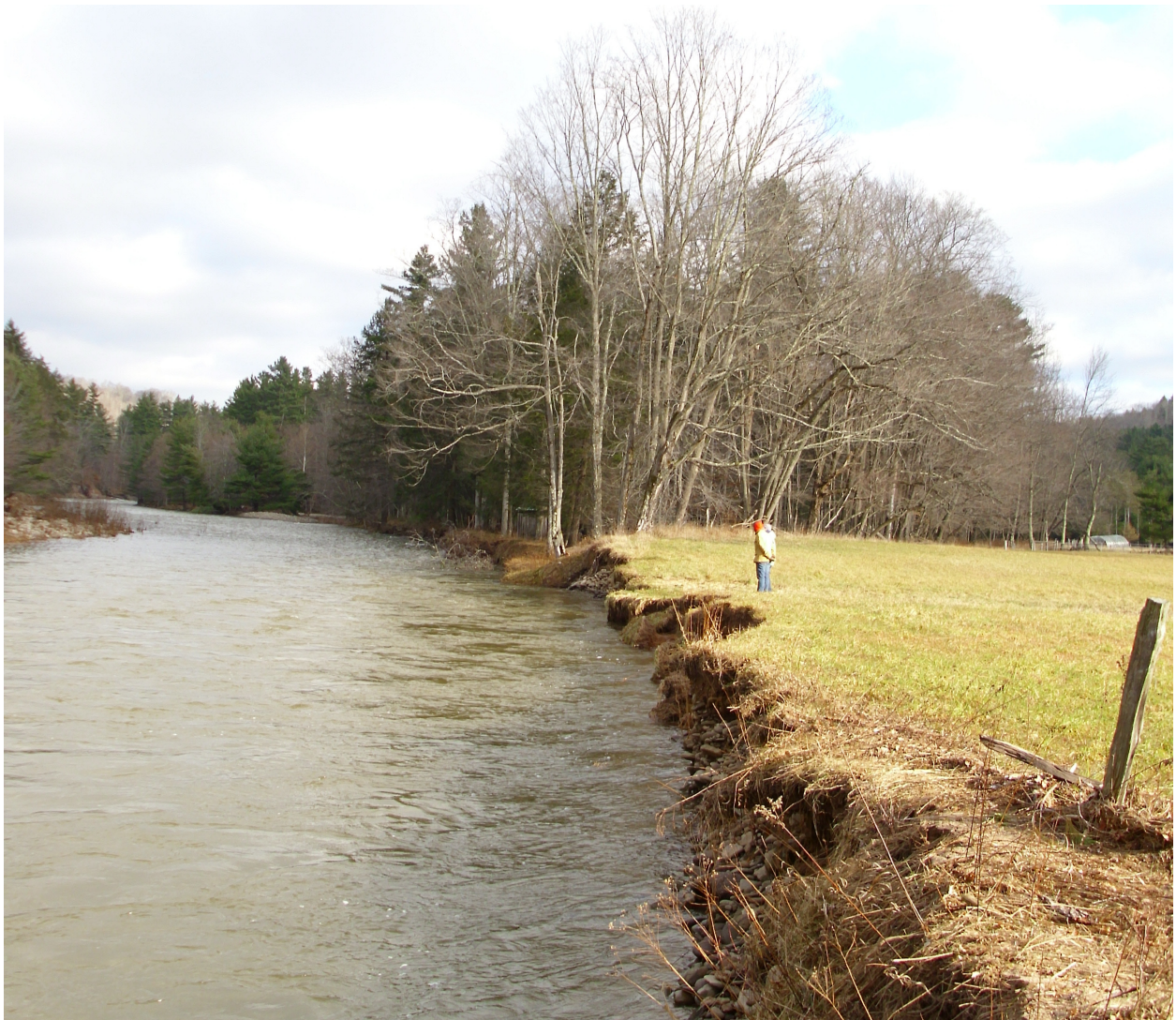
Streambank with no vegetated buffer protection. (DSCI0318)
