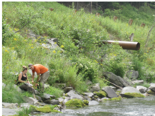
Piped outfall and rip-rap on left bank adjacent to Claryville Road (B479)
