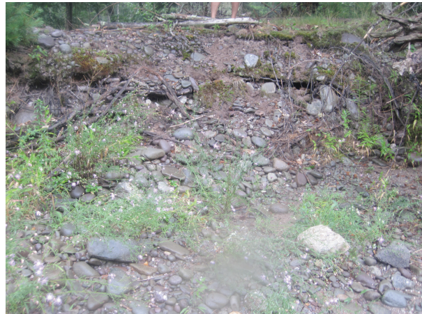
Sedge and alluvial material at right bank erosion point (A176)
