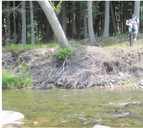
Scour and undercutting on right bank (A321)
