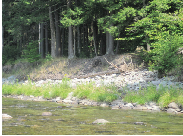
Erosion on right bank (A318)
