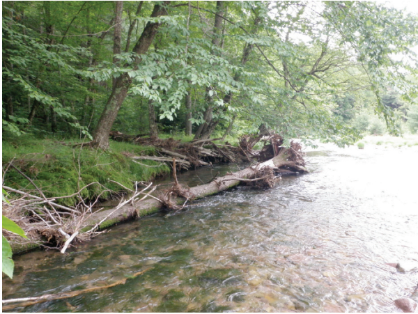
Large tree deposited along left bank (B226)
