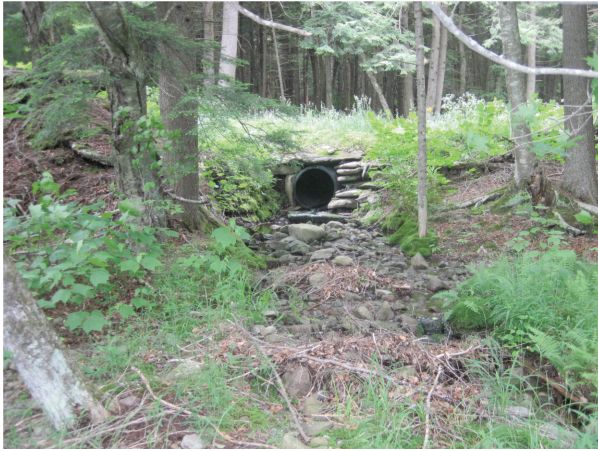
Small tributary entering on right bank through culvert under Denning Road (A334)
