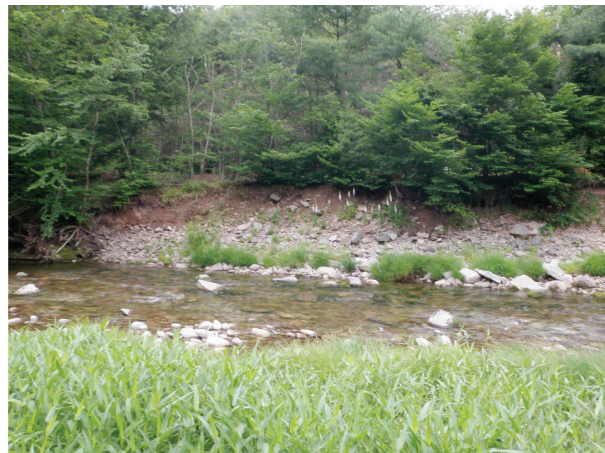
Erosion on right bank due to hydraulic pressure (B224)
