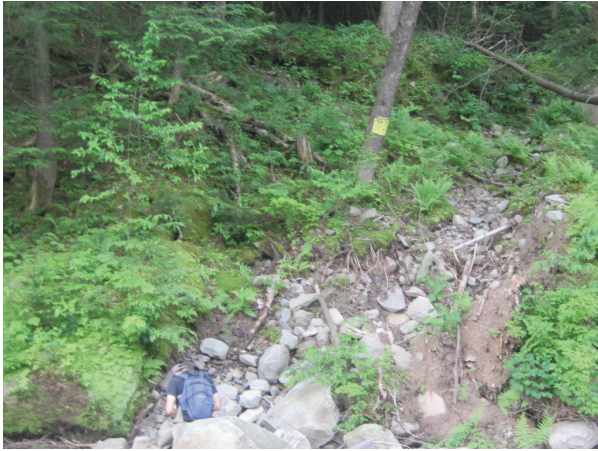
(B224) Hydraulic erosion on left bank
