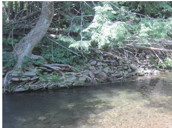
(B249) Hydraulic erosion downstream of revetment
