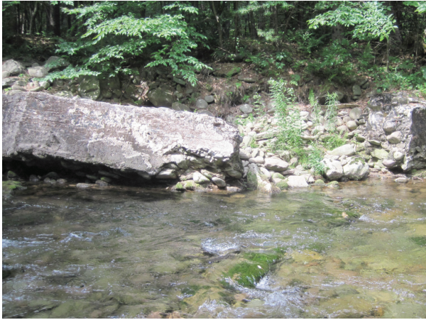
(B244) Crumbled bridge abutment serving as revetment
