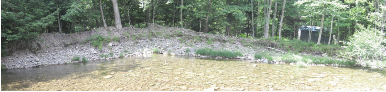
(B251-253) Severe hydraulic erosion on left bank
