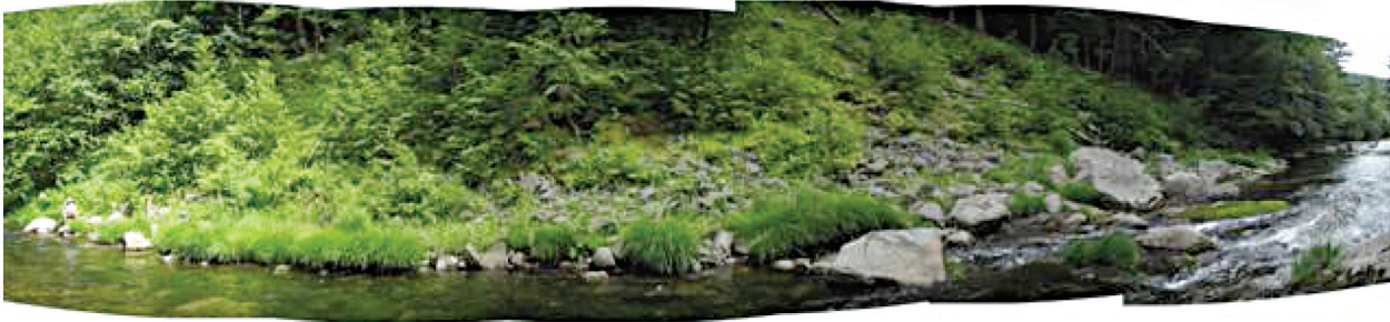
Naturally repaired left bank failure (A210-215)
