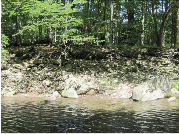
Erosion on left bank (B319)
