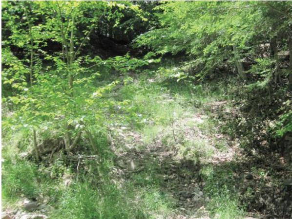
Slope failure due to upland drainage (A358)
