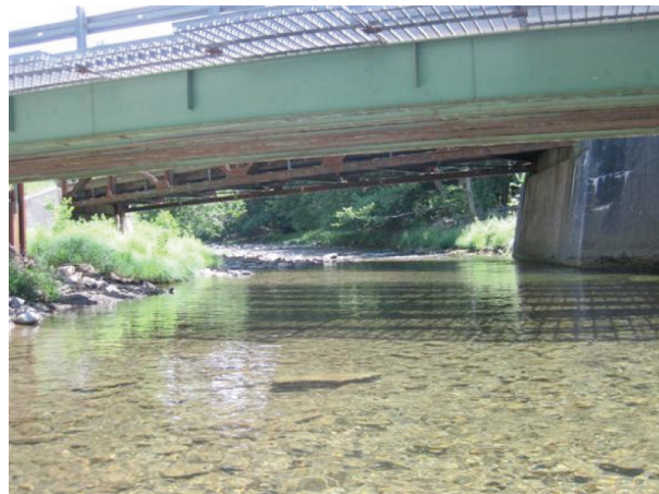
Aggradation under bridge (A326)
