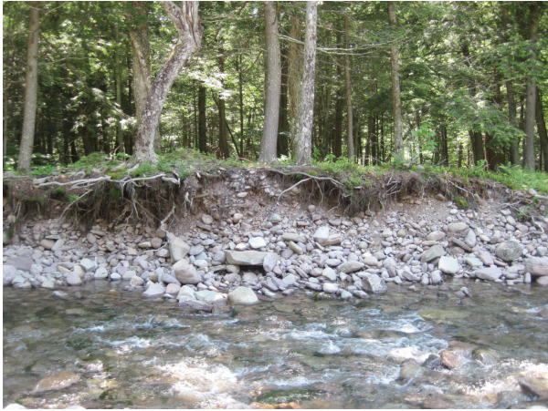
Right bank erosion showing unconsolidated alluvial sediments (A43)
