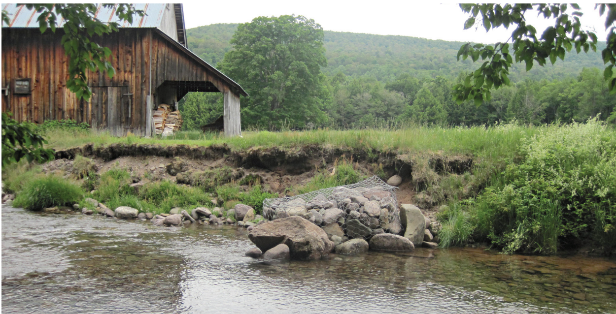
Erosion on right bank (A83)
