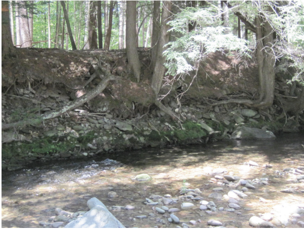
Erosion along right bank (B407)
