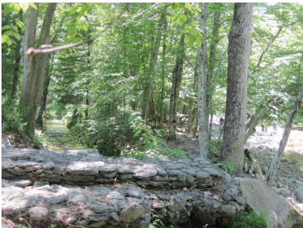
Gabion baskets preventing scour caused by divergence (A526)
