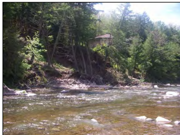
Bank erosion at 78900
