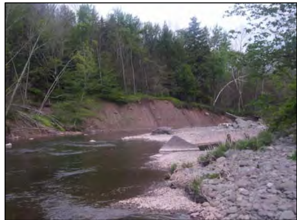
Bank erosion at Station 89670
