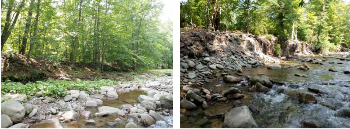
Figure 22 Berm, Stn 100-500, left bank; Erosion, Stns 160-350, right bank
