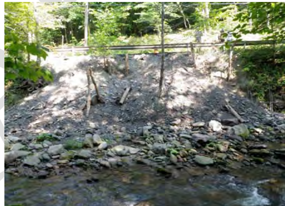
Figure 7 Bank erosion, right, Stn 3200, ungraded dumped fill
