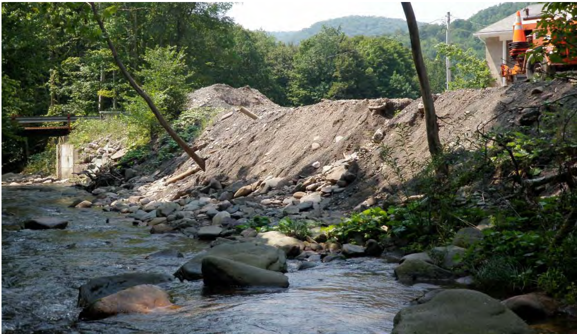
Figure 17 Eroding bank adjacent to Ulster County Highway Garage yard
