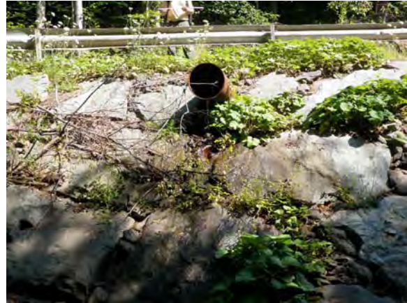
Figure 6 A smooth steel piped outfall causing some scour on the right bank
