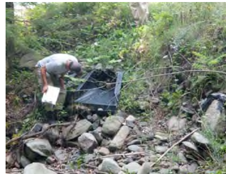
Figure 18 A highway department storm water retention pond drain on the right bank
