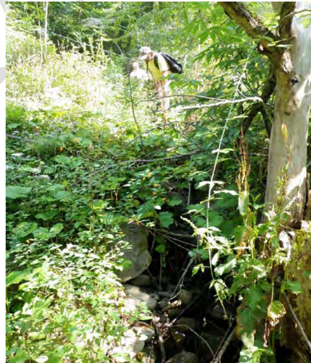
Figure 11 Smooth steel culvert outfall, undermined by soil piping beneath pipe
