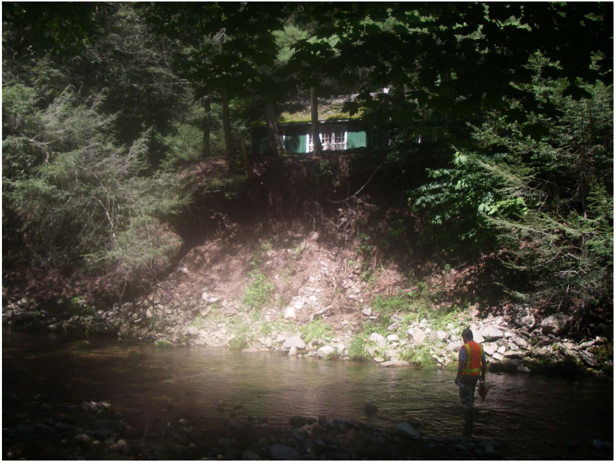
Figure 6 Erosion at Stn 22000, right bank
