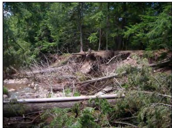
Erosion along right stream bank Stations 69616-69400
