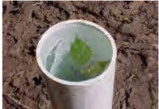
Photo 11. Groundwater relief well on the failing hillslope during construction, showing water from 30 feet down flowing up out of the ground under pressure. Note groundwater is clear before it comes in contact with the clay layers.
