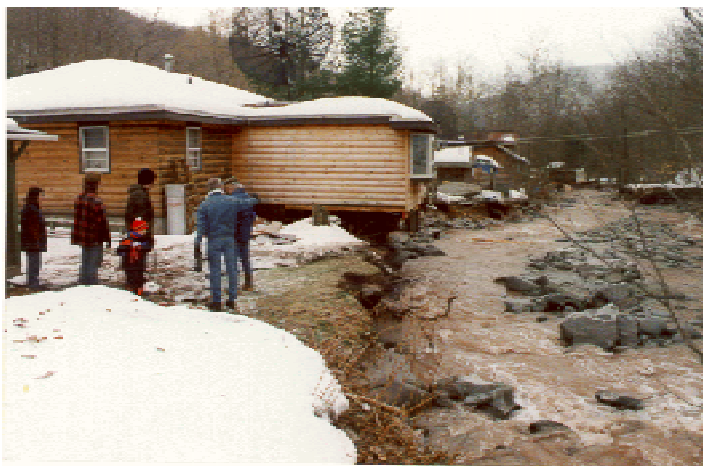
Photo 2. Looking downstream at left bank eroded under the Torregrossa home, 1996, following the January flood event.
