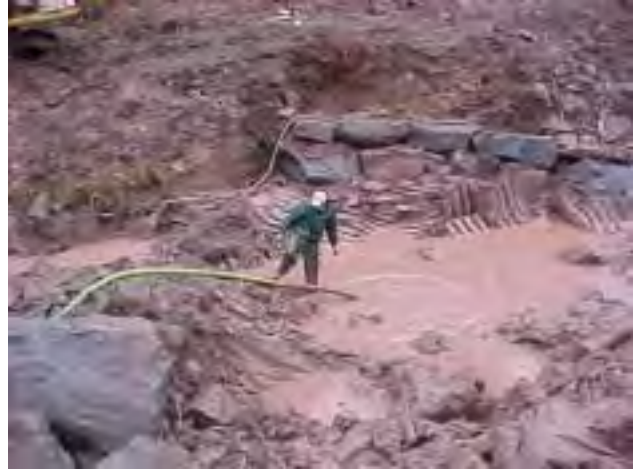
Photo 12. Excavation of a plunge pool below a cross vane during construction, 2000. Clay material in the stream bed was over-excavated and removed, and back filled with clean sediment to form the new stream bed.
