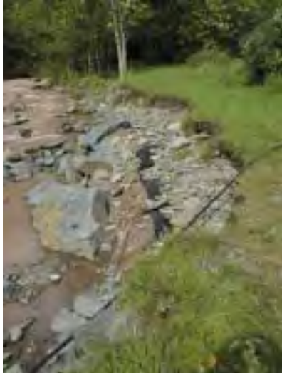
Photo 4. Looking upstream, failing rip-rap along left bank opposite clay hillslope, mid-MU3, 1998.
