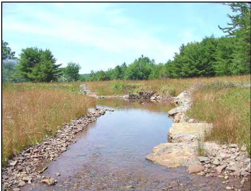
Figure VII-20: View of completed Big Hollow reach less than one year after construction.
