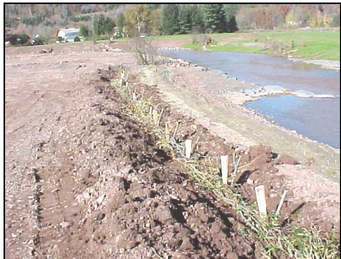
Figure VII-7: Rows of willow fascines are planted on meander bends to provide vegetative protection.
