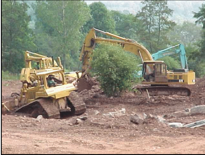
Figure VII-14: Heavy equipment working to construct the design channel at the Brandywine site.
