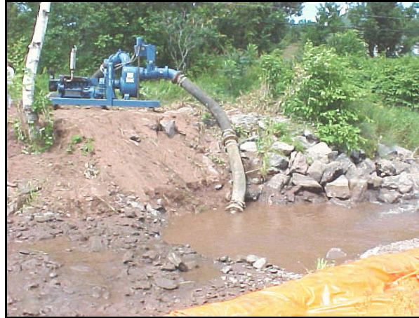
Figure VII-3: A 12" diesel pump was used to intercept and pump around all upstream flow entering the project site.
