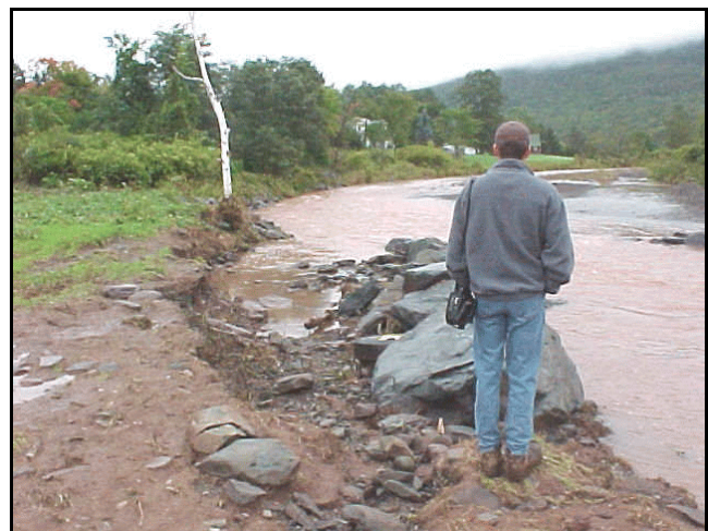
Figure VII-23: Scour behind Cross Vane arm due to loss of depositional feature attributed to voids between vane rocks
