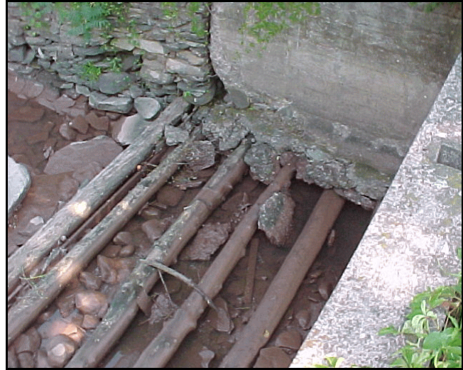
Figure VI-59: Invert of right bridge opening. The hemlock logs had been covered by concrete.
