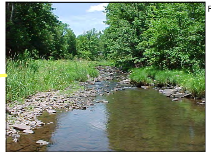
Private bridge exhibits good stability, and does not appear to be impacting the stream
