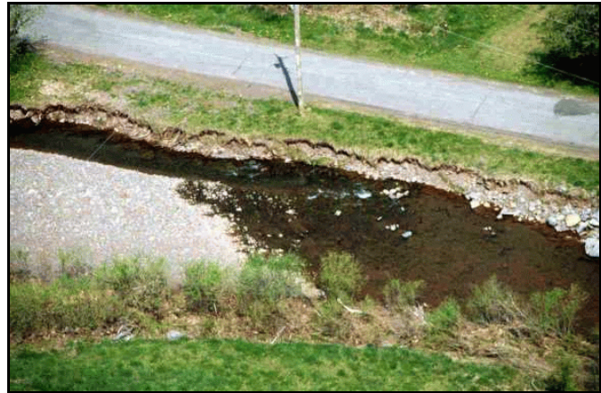
Figure VI-8: Aerial view of lateral migration along County Route 56 in lower section of management segment 1b.
